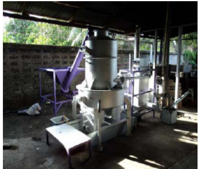
Fig. 4: configuration of the gasifier system used
