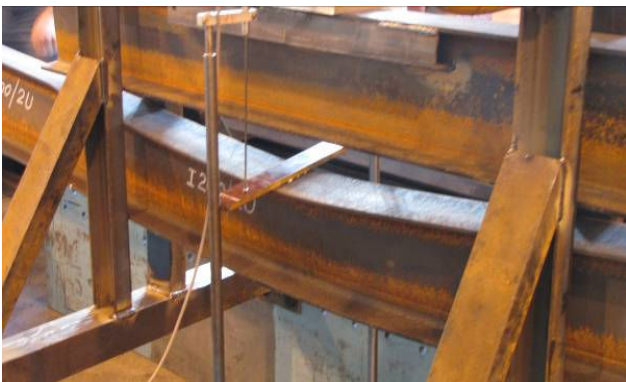
Fig. 7 typical failure of CFRP strengthened steel beam
